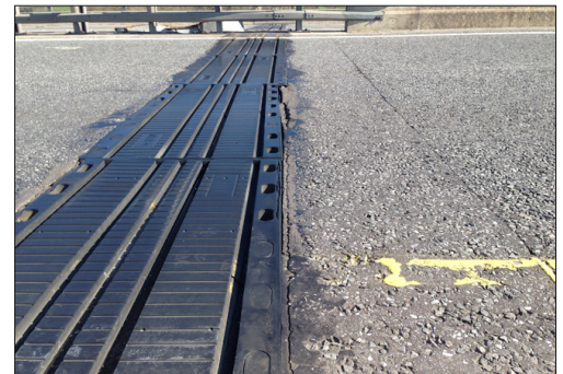
Failed expansion joint - showing detachment from surface, delamination and joint exposure.
