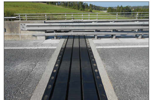
New installed TF1300 expansion joint
