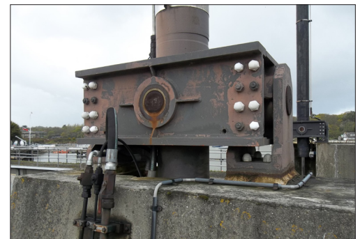
Fishbourne Ferry Port - Condition of existing gimbal showing wear and corrosion
