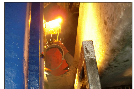
Portsmouth Ferry Port - Underside burning of bolts to release cylinder ready for removal
